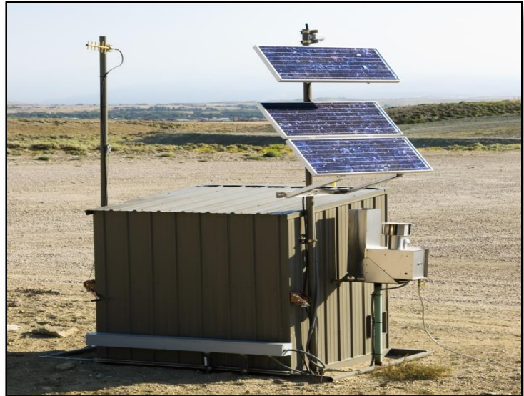
Wireless communication equipment deployed at an oil field pump-jack site.
